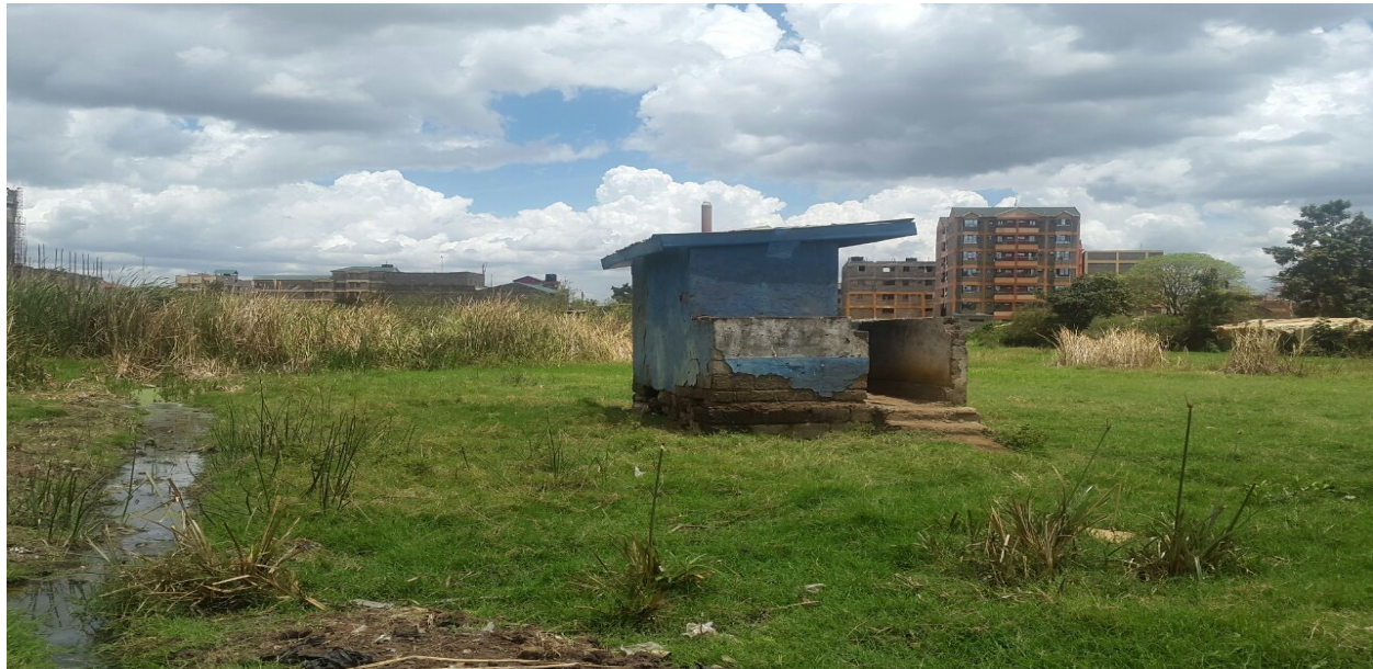
Plate 4: Dilapidated Toilets in Juja Market
