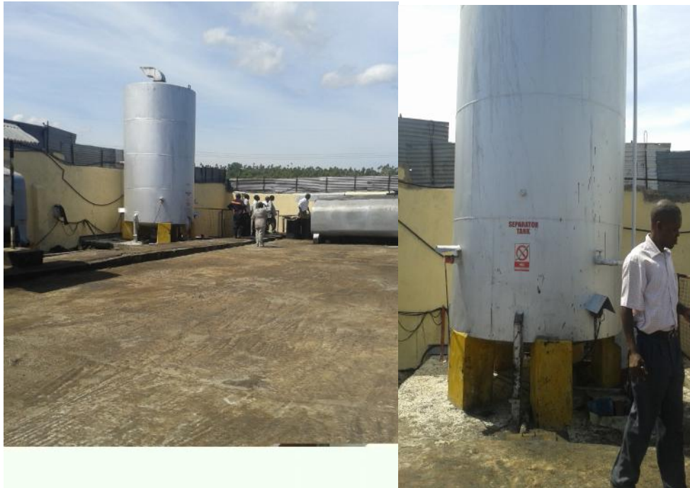
Plate 10: View of an oil and water separator tank at a facility
