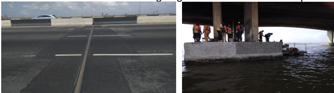
Picture 14: Part of the Completed Expansion Joints and Repair of Pile Caps in Progress at the 3 rd Mainland Bridge, Lagos
