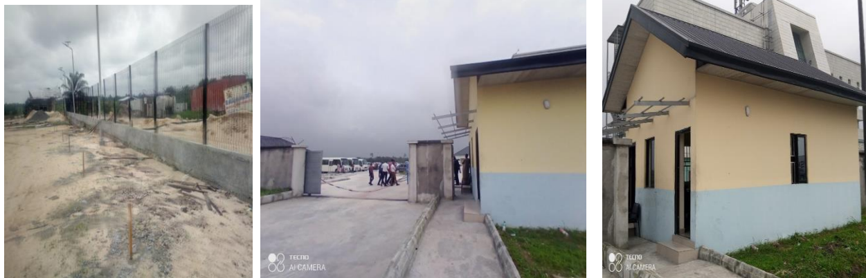
Picture 72: Completed Sand Filling, Gate House and Access Road at OGFZA, Onne Port Harcourt
