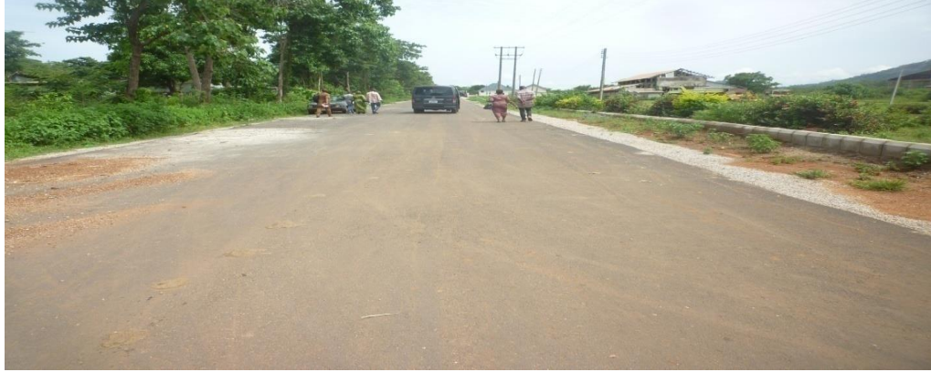
Picture 76: The Ongoing Rehabilitation of Internal Road at Iron Ore Mining, Lokoja
