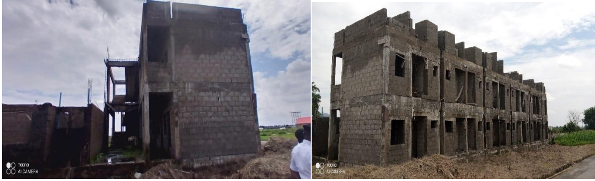
Pictures 56: Ongoing Construction of 1No. L-Shape Female Hostel Accommodation at National Fire Service Academy, Sheda
