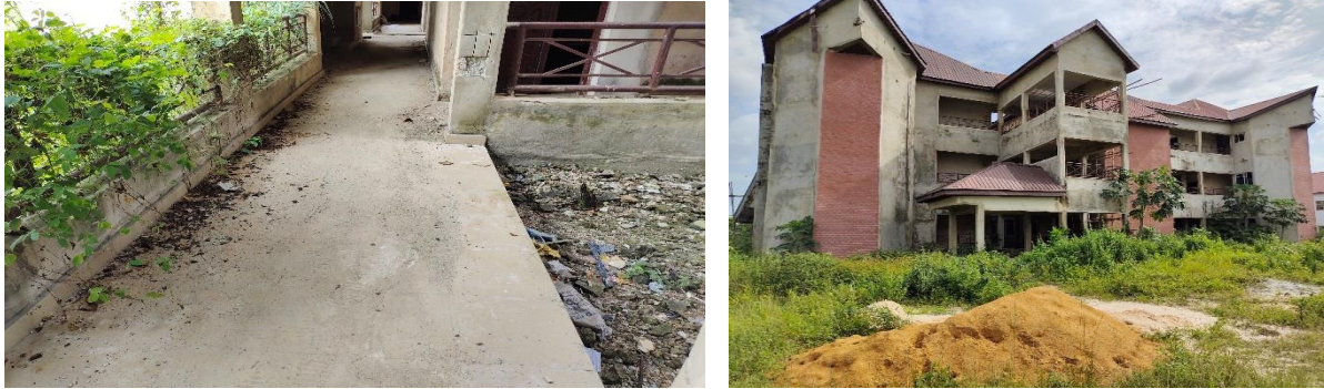
Picture 50: Ongoing Construction of School of Science Complex Phase I at the Federal University of Technology, Owerri
