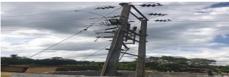
Picture 30: Part of the Biakpan Electrification Project at Biase Local Government Area in Cross River State
