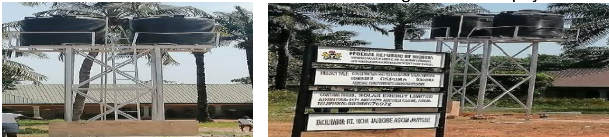
Picture 79: Constructed Solar Powered Borehole in Ogoja and Yala of Cross River State
