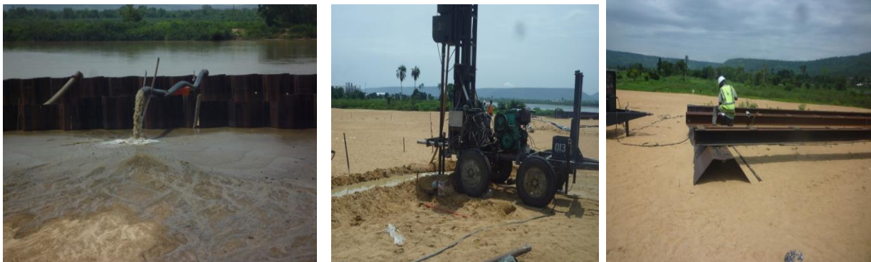
Picture 63: Ongoing Casing of Steel Bins for Foundation of the Transit Shed and Drilling of Foundation Pile at NIWA
