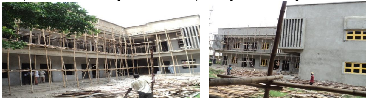
Picture 62: Ongoing Construction of 4Nos. Blocks of Classrooms, Laboratories and Twin Theatres at NITT, Zaria
