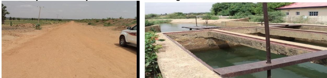
Picture 21: Part of the Rehabilitated Service Road and Water Intake at the Main Canal
