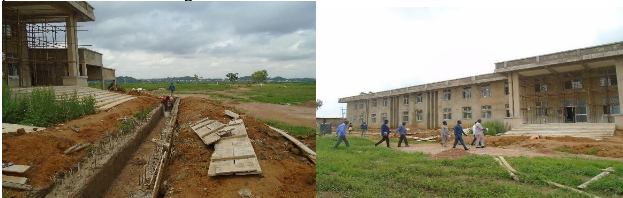
Picture 40: Ongoing Construction of Additional Ward (Amenity) at the Jos University Teaching Hospital, Jos
