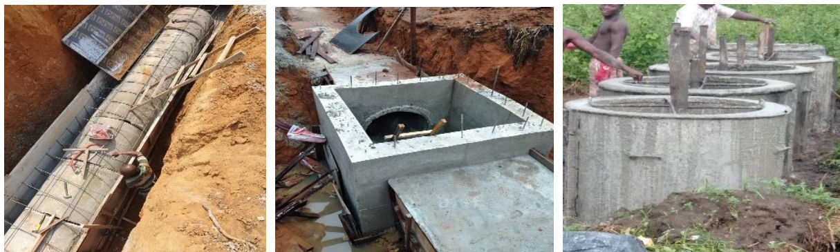
Picture 73: Completed Construction of Underground Drainage Extension to Discharge Point – IITA Road, Onne, Port Harcourt
