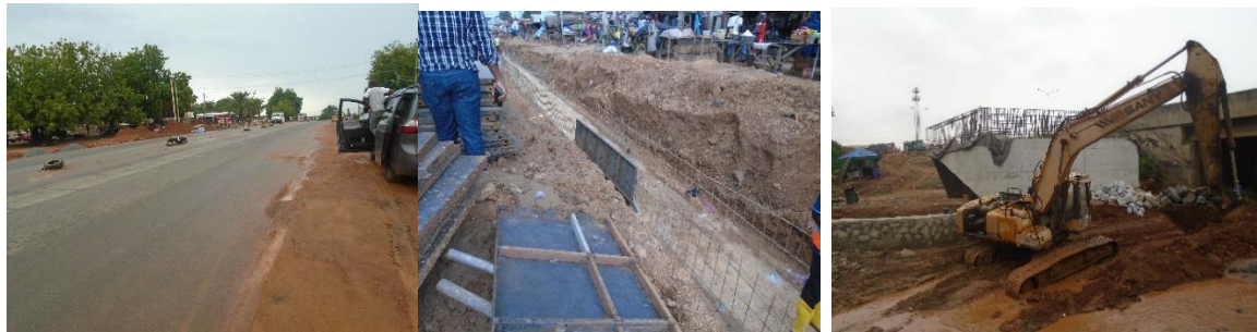
Picture 10: Ongoing Asphaltic and Bridge Works at Abuja – Keffi Sections of the Road.
