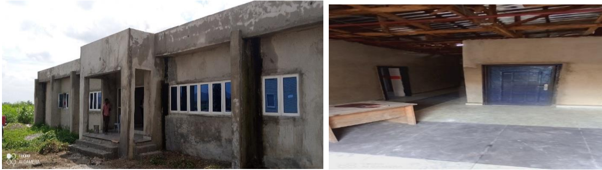
Pictures 54: Ongoing Construction of BA Refiling Plant Abuja/Design and Construction of 1No. BA Gallery
