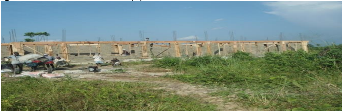
Picture 68: Ongoing Construction Work of Academic Research and Training Building at Osubi Campus PTI, Effurun.
