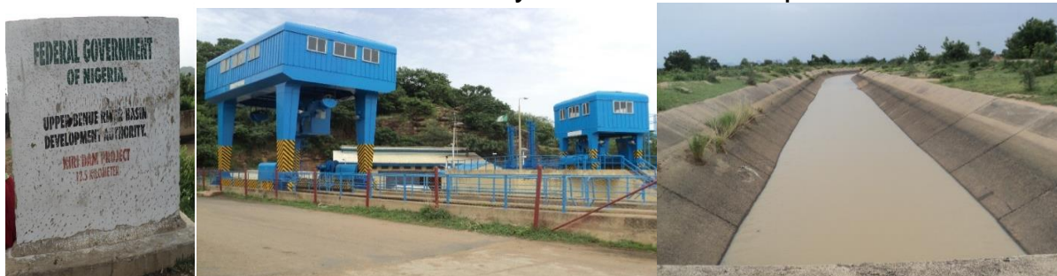
Picture 22: Completed Maintained Work of Gantry and the Rehabilitated Conveyance Canal at Kiri Dam Irrigation
