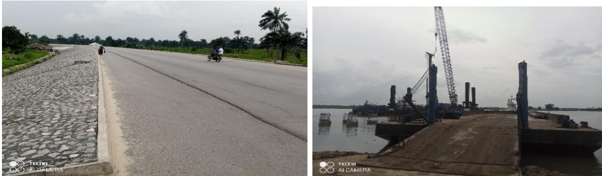
Picture 9: Ongoing Construction of Bodo – Bonny Road with Bridges Across the Opobo Channel Route in Rivers State
