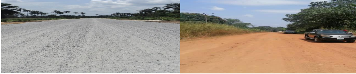
Picture 78: Completed Section of the Asphaltic Top Coat Rural Mining Road and Ongoing Substantially Portion in Ibil Community of Cross River State
