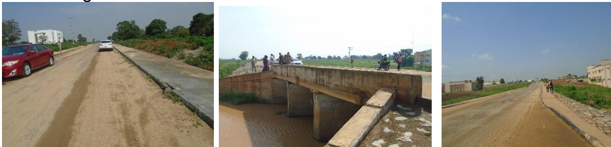
Picture 45: Completed Triple Cell Culvert and some Portions of Road at the Federal University, Lafia
