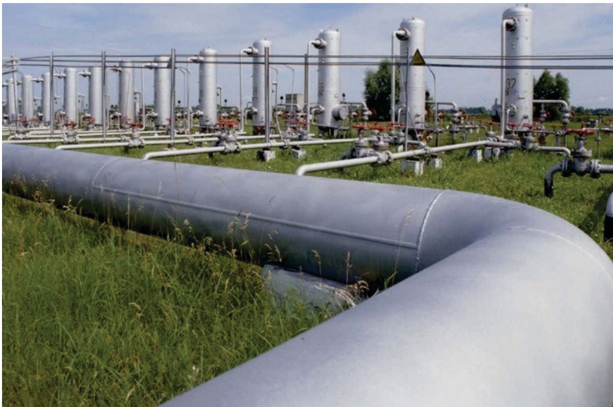
■ Oil Pipeline in Nigeria
