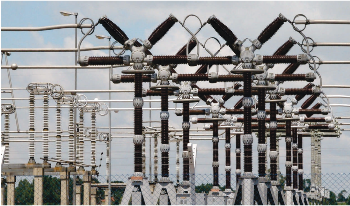
■ Power Sub-Station, Abuja.
