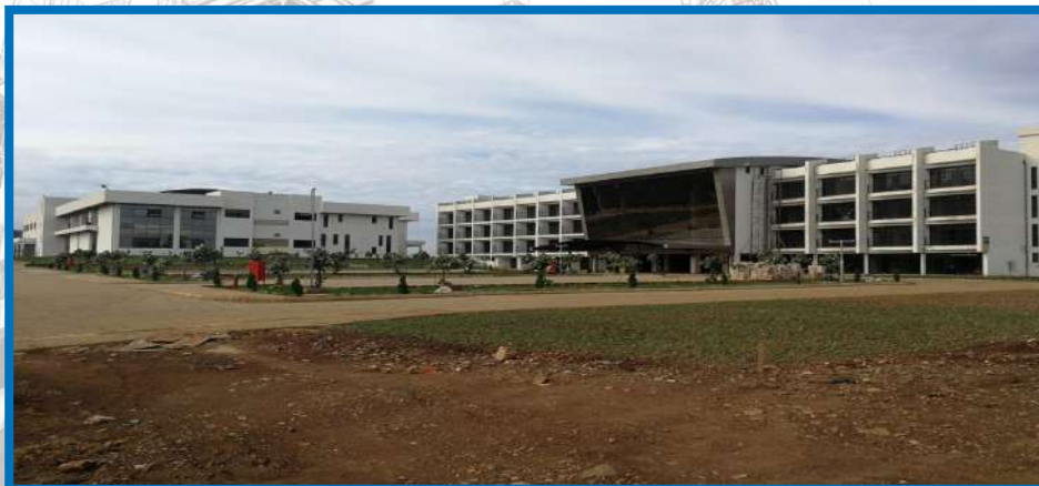
Construction and Finishing Works for Kivu Marina Bay 4 Star Hotel in Rusizi
