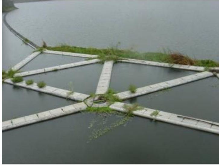
Figure 0.9 KGPS water intake screen (photo)
